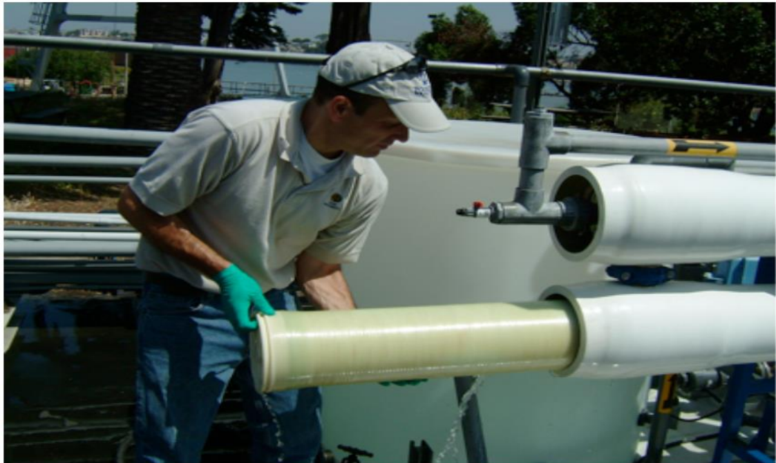
Figure 1 – RO membranes – the “work horse” of today’s desalination plants
